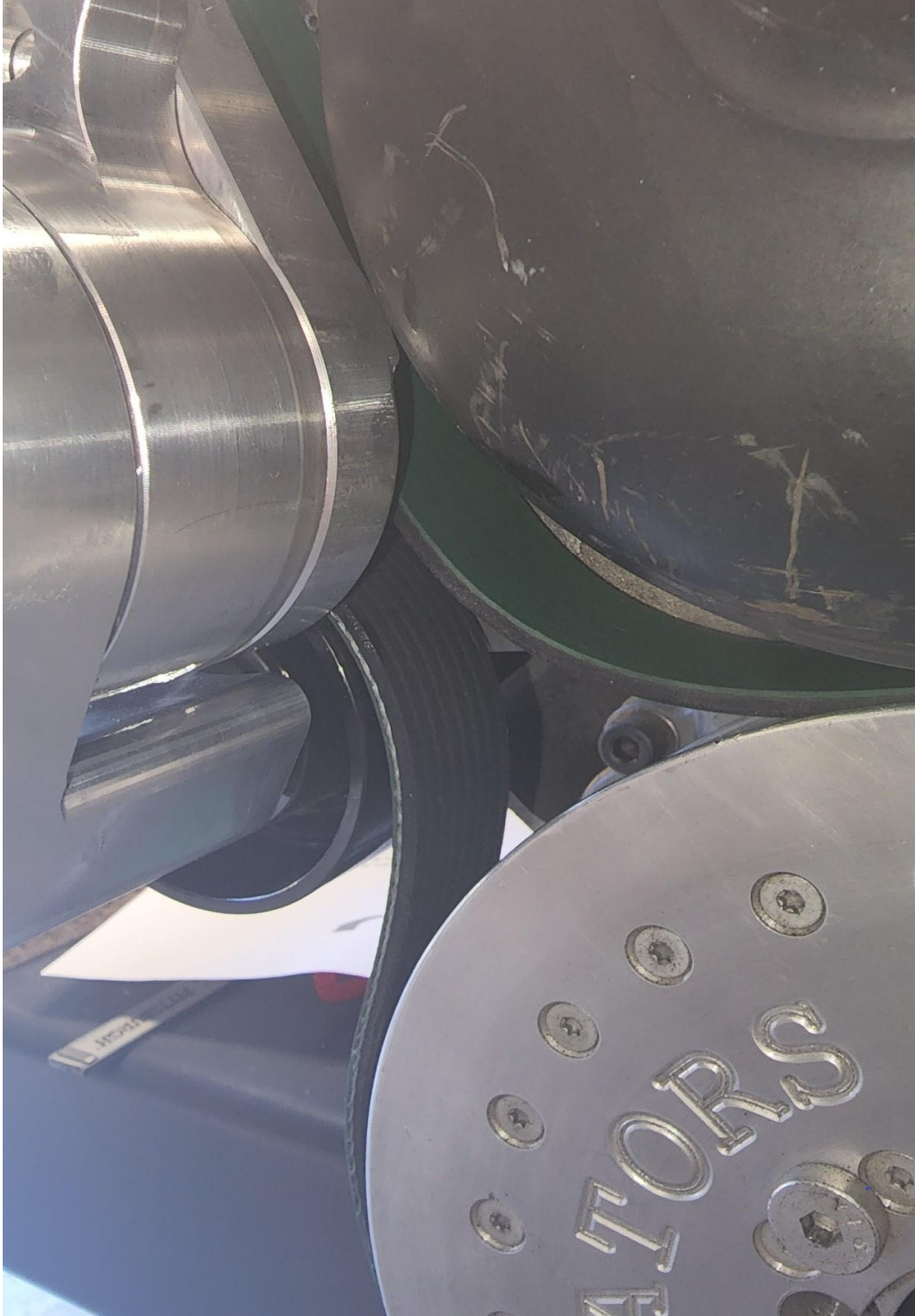
BELT COMING OFF TENSIONER AND UNDER BALANCER
