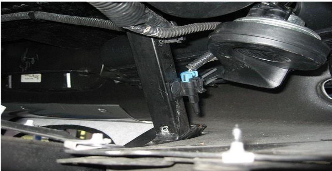
TEMP SENSOR MOUNTED
